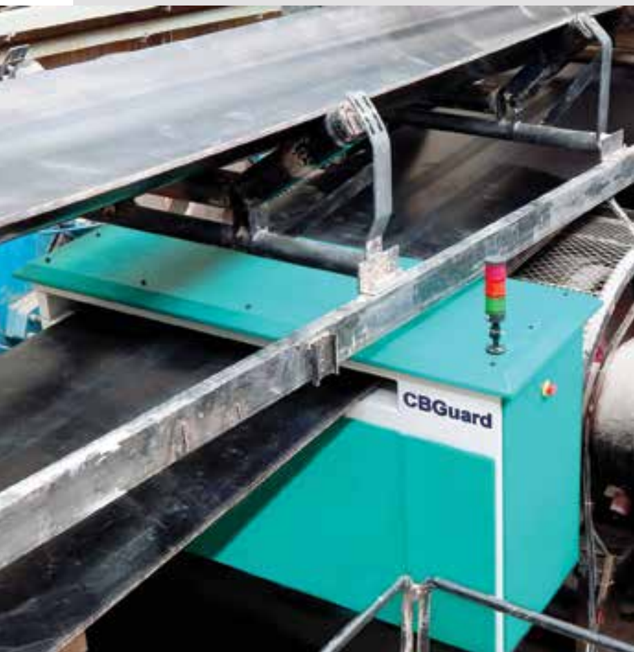
CBGuard system in place on a conveyor.
